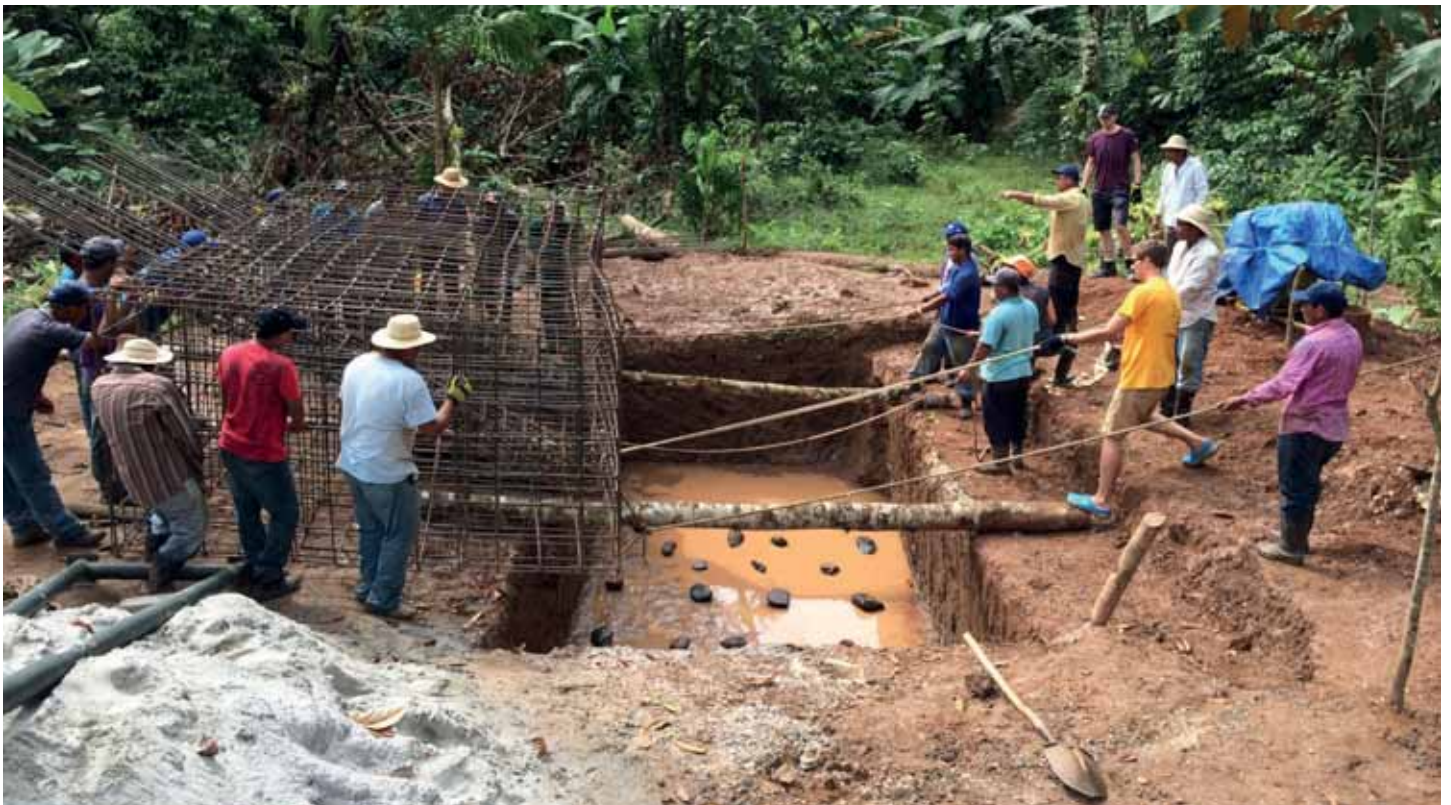
↑ Water in ankerbloksparing
