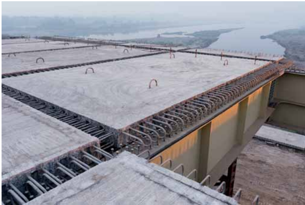
Steel grid with precast concrete panels on top before closing of the joints. © Andreas Deffner
