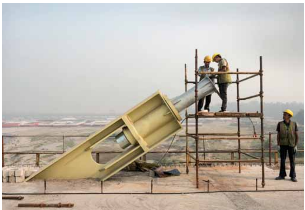
Passive cable anchorage at deck level. © Andreas Deffner
